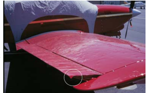
Figure 8: Hail damage to wing skin of a general aviation aircraft parked at the Front Range Airport (KFTG).
